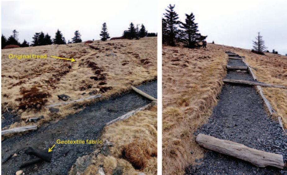
Figure 6. Restoration of a steep “fall-line” segment of the Appalachian Trail (left) in the popular Roan Highlands area of North Carolina. Restoration work conducted in 2001 included laying native sod excavated from the new side-hill alignment (right) and temporary fencing to discourage use. Geotextile fabric and cellular confinement materials were used, but both surfaced after displacement of the applied gravel. Premixing gravel with native soils is a more natural and sustainable practice.
